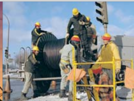
Low- and Medium-Voltage Distribution Cables
