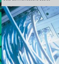
Data Communications Cables
